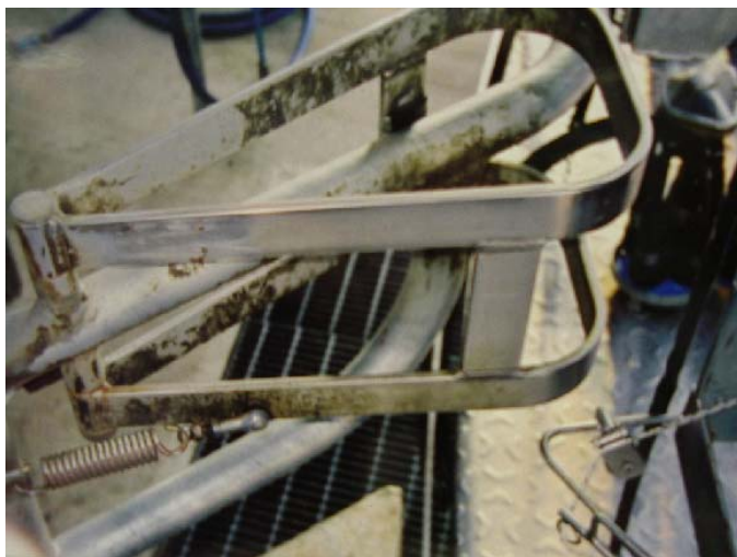
Typical entry safety switch
