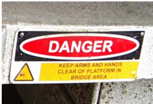
Warning signs required at pinch points between platform and bridge.
