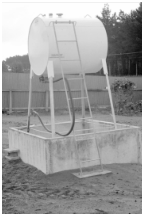
Example of a compound to contain fuel if a leakage or spillage occurs.
