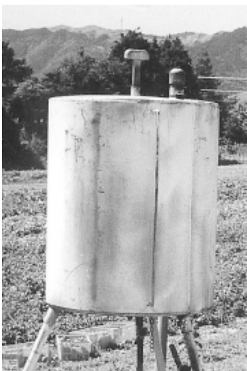
Tanks shall be of sound construction, with no serious corrosion.
