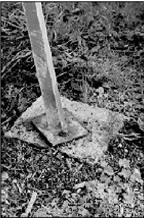
The feet of a tank should not be buried as this can lead to rapid corrosion, and their condition cannot be checked.
